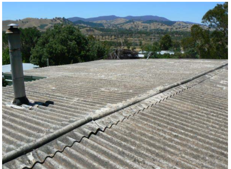
Before shots – cracked asbestos roof
